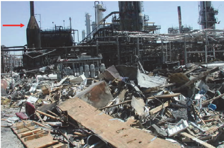
Figure 2.3. Destroyed trailers west of the blowdown drum (CSB 2007)
