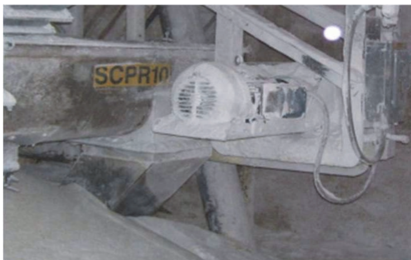
Figure 4.4. Motor cooling fins and fan guard with sugar dust, piles of sugar on floor (CSB 2009)
