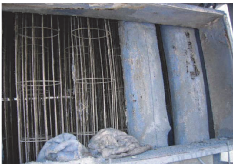
Figure 11.18. Damage to dust collector bags (Garland)
