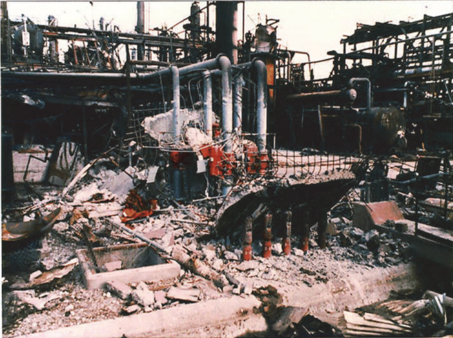
Figure 15.1. Oxidation reactor after explosion (Celanese)
