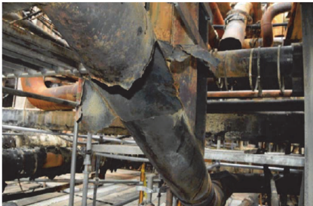
Figure 11.36. Piping rupture (CSB 2015)
