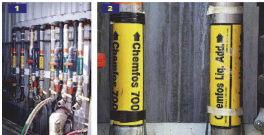
Figure 11.29 1 - Pipe connections in panel 2 and Chemfos 700; 2 - Liq. Add lines (CCPS f)
