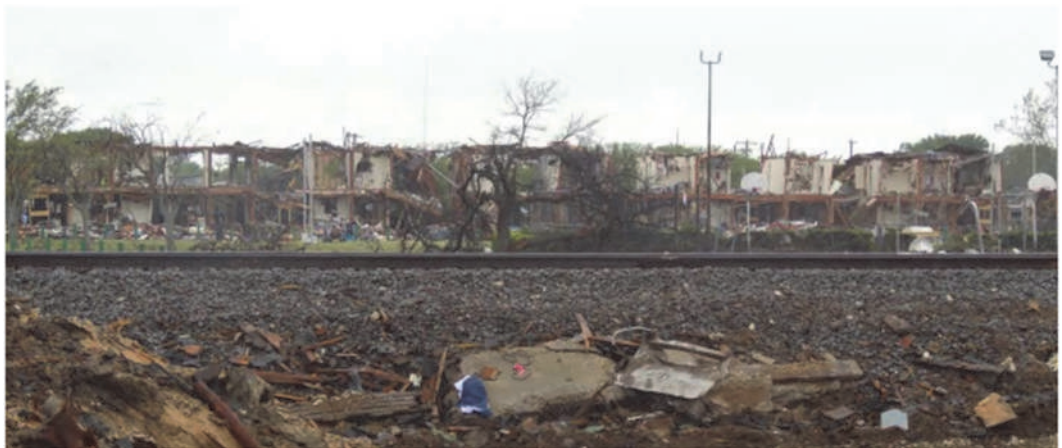
Figure 20.5. Apartment complex damage (CSB 2013)
