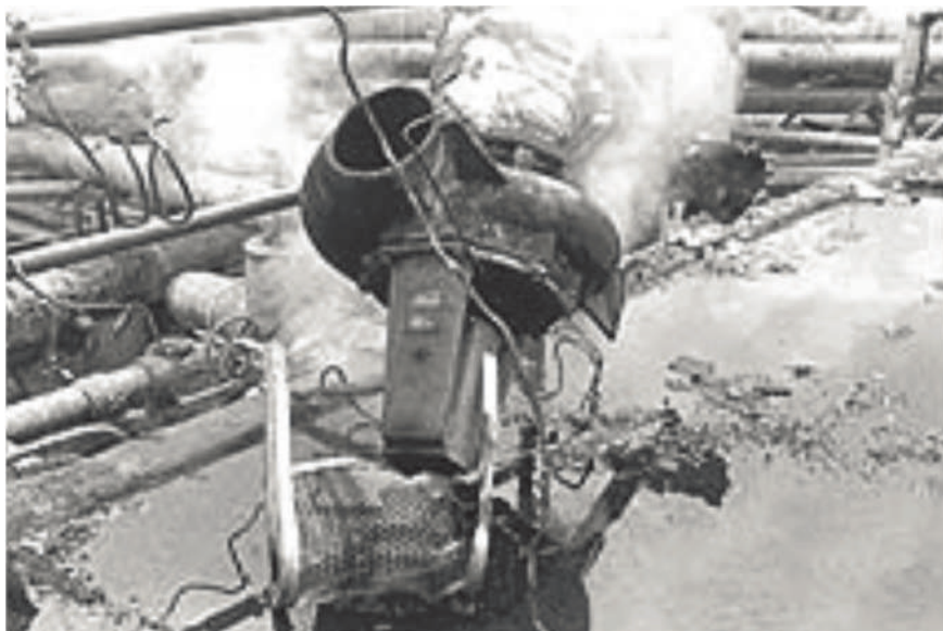
Figure 11.6. Pump explosion from running isolated (CCPS 2002 b)
