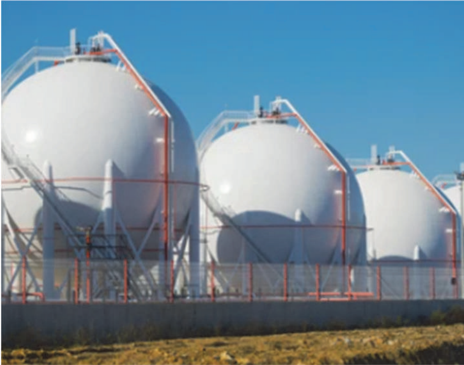
Figure 11.35. Pressurized gas storage tank (shutterstock)
