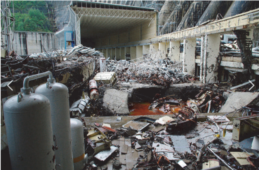
Figure 8.4. Damage in the generator hall at the Sayano-Shusenskaya hydroelectric plant (AP)
