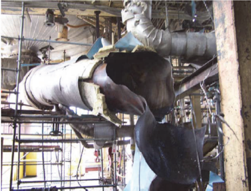
Figure 11.12. Ruptured pipe from reaction with heat transfer fluid (CCPS h)
